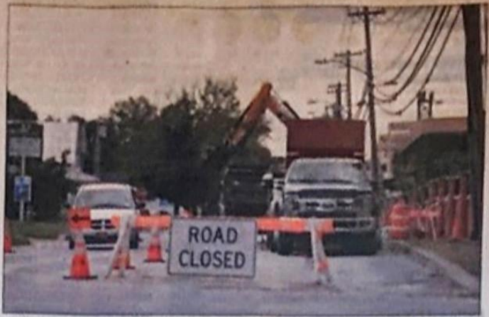
A road closed sign sits in front of road construction crews as they begin work on Boynton Avenue in Plattsburgh. Boynton Avenue was the next scheduled street to be worked on, followed by Clinton and Steltzer streets, after the repaving of sections of Cornelia and South Catherine streets.
